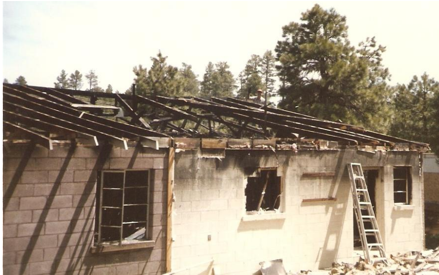
Fire damaged home
