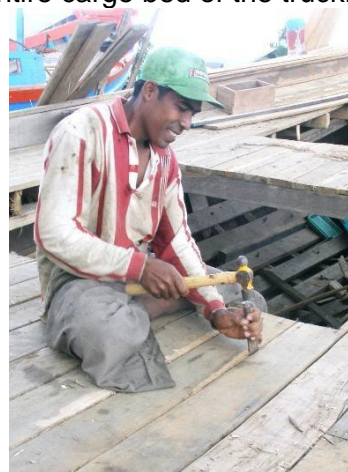
A craftsman sealing the seems in the decking of the Islamic Relief boat.
