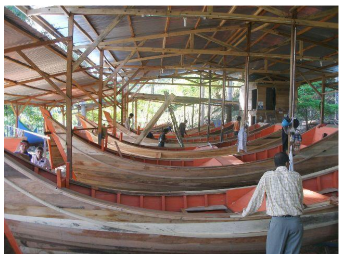
The Krueng Raya boat yard with ten boats under construction at one time
