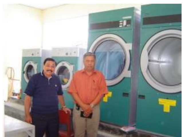
new commercial grade washers and dryers with member-specialists who helped install and assure proper operating capacity
