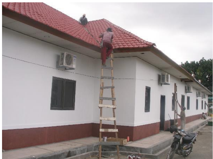
The former building was completely renovated and remodeled. These workers are installing a new roof and air conditioning units.
