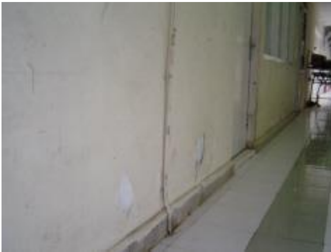
Mental hospital condition after tsunami water damage
