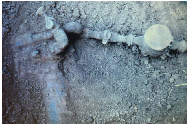
Likely Mountain Dell connection to pipeline
